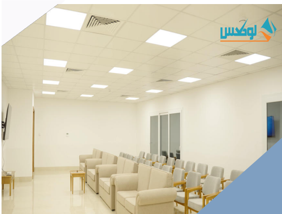
Interior & Exterior lights at RCA accommodation - Muscat - 2026
