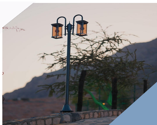
Pathway lighting at Mountain walk road-Nakhal- 2025
