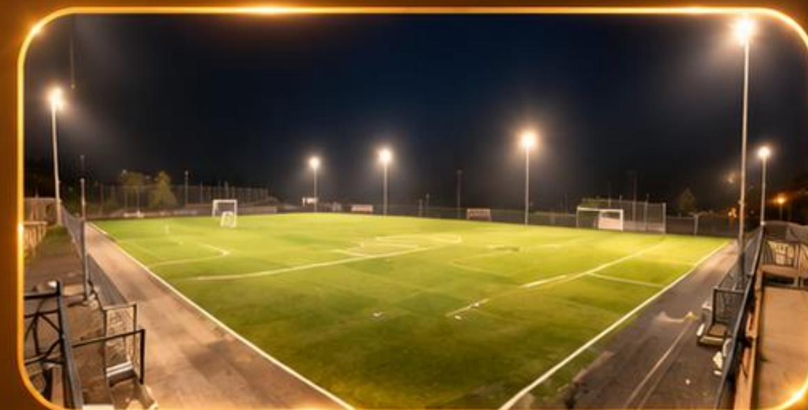
HIGH MAST LIGHTING
