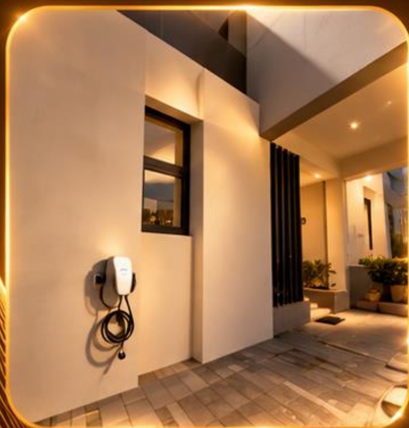
ELECTRIC VEHICLE CHARGER
